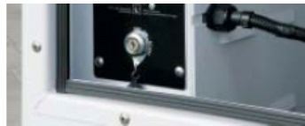
Engine control panel with emergency shutdowns
